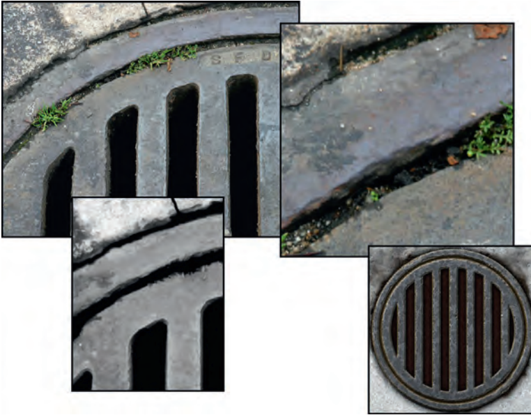
FIG 1.33 This sewer intrigued me: a simple shape of a common item that many might overlook as not worthy of serious attention. Some may have the attitude that it is only a sewer grate, so make it and move on. But a shiny new sewer grate with clean edges would stand out in a grungy urban setting. Look at this sewer grate. It is made of iron and looks solid and heavy. It was probably laid down decades ago and has had thousands of cars drive over it, people walk over it, millions of gallons of rainwater pour through it. On the image at the upper left you can look at the iron and see how it is rusted, but it's so well worn that the rust is polished off in most places. Dirt has built up in the cracks between the grate, the rim, and the concrete. Even little plants have managed to grow. Look at the close-up at the upper right and you can see just how beat-up this iron is and how discolored it has become. At the lower left, I desaturated and cleaned up a portion of the image to see just how the light and shadow are hitting it and to get a feel for the quality of the surface. In this image, you can more clearly see the roughness of the cement and the metal, and although the circular grate looks round from a distance, up close there are no straight edges and smooth curves. All this detail can't be depicted 100% in a game texture, but knowing it's there and understanding what you are seeing will allow you to convey a richer version of the grate as you learn to focus on those details that add realism and character. On the lower right is a texture I did, and you can see that I was able to quickly achieve a mottled and grungy look for the metal and the edges. There are a few places at the top where I started the process of eating away at the concrete and the metal a bit.
